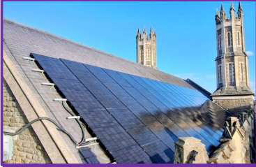
Solar Panels and Batteries
