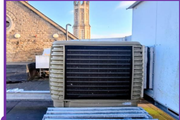
Air Cooler System—prayer hall
