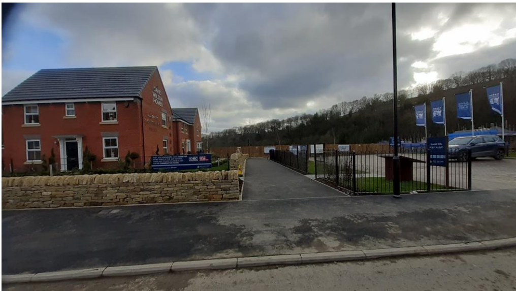
The first few meters of the UDT have now been built at Oughtibridge Valley
