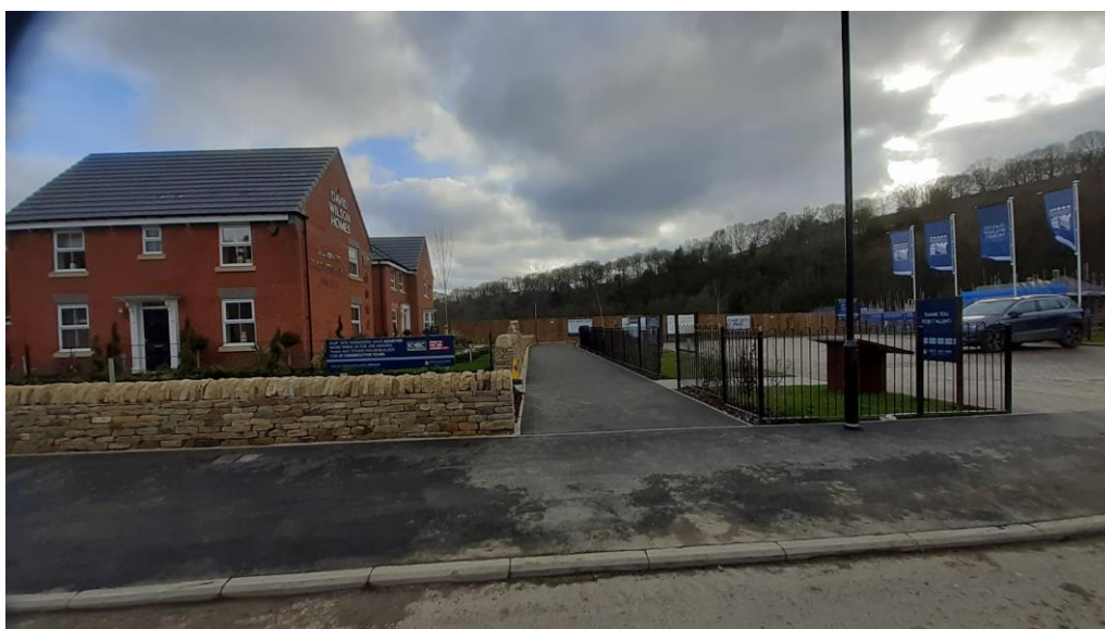
The first few meters of the UDT have now been built at Oughtibridge Valley
