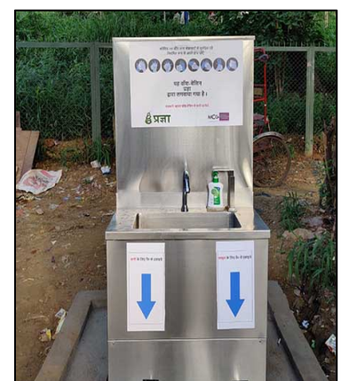
A foot pedal operated handwash station installed by Pragma
