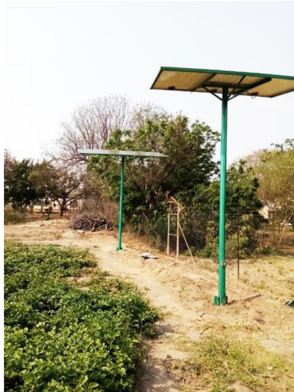
Solar panels to power water pump
