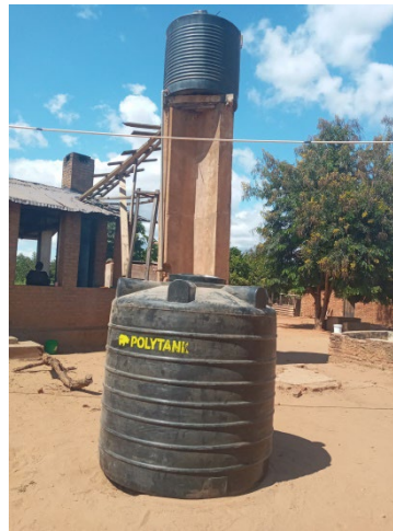
New distribution tank
