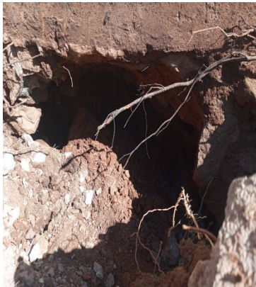
Scour under the main tank
